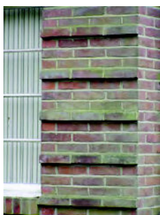
Picture 9.25 Projecting bricks
