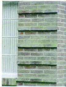
Picture 9.25 Projecting bricks
